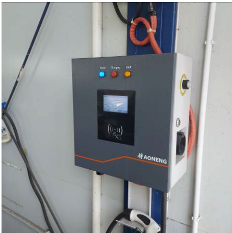
22 kW AC charging facility
